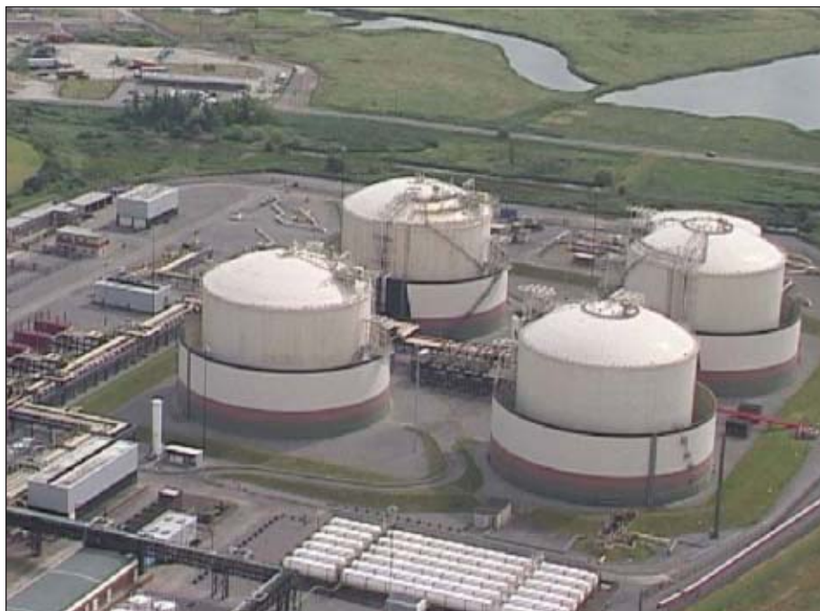
UK's Isle of Grain LNG terminal began operations in July 2005 and has current capacity of 3.3 million tonnes/year (Fig. 2; photo from Grain LNG).
