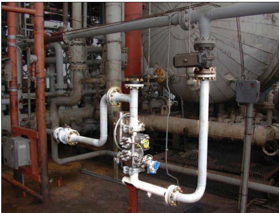
Perenco installed permanent PhaseWatcher Vx29 multiphase meters on the Yombo platforms (Fig. 6).
