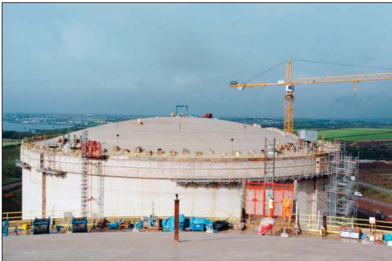
Construction progresses on one of two 168,000 cu m storage tanks at the Dragon LNG terminal, Milford Haven, UK. The 4.4 million tonne/year terminal is set to begin operations later this year and could expand to 6.6 tpy in the near future. Photograph from Dragon LNG, BG Group.
