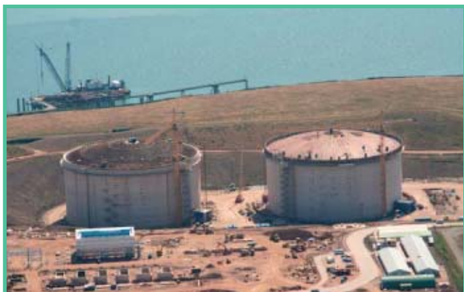
Tanks for the Dragon LNG terminal, Milford Haven, UK, near completion earlier this year in preparation for terminal start-up in late 2007 or early 2008. Each tank will be able to store 168,000 cu m. The terminal will initially accommodate 4.4 million tonnes/year with plans to expand to 6.6 tpy in the near future. Photograph from Dragon LNG, BG Group.
